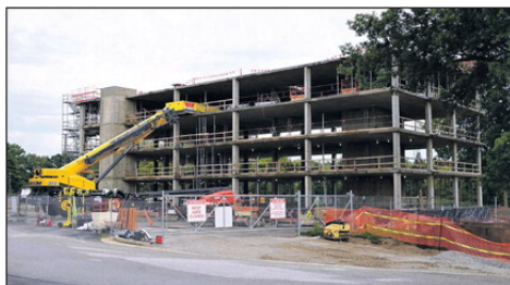
A new Rose-Hulman Institute of Technology residence hall, seen here on Thursday, is the first new freshmen residence hall to be built since 1962. The four-story, $30 million structure will be ready for occupancy in fall 2025.
